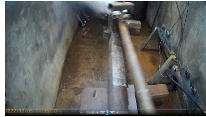
Y7 pipeline section
