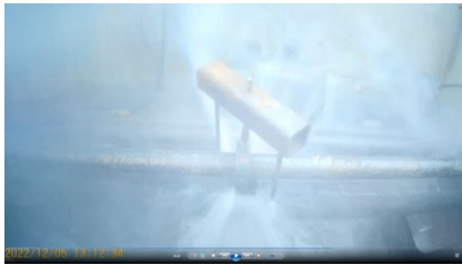
Y8 pipeline section
