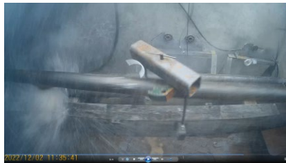
Y10 pipeline section
